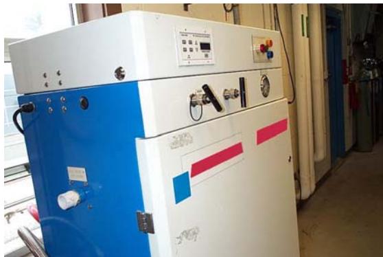
NEA Machine to produce N2
