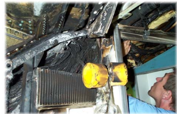
Fire in Bulkhead AirTran DC-9-32, Greensboro, 8/8/00
