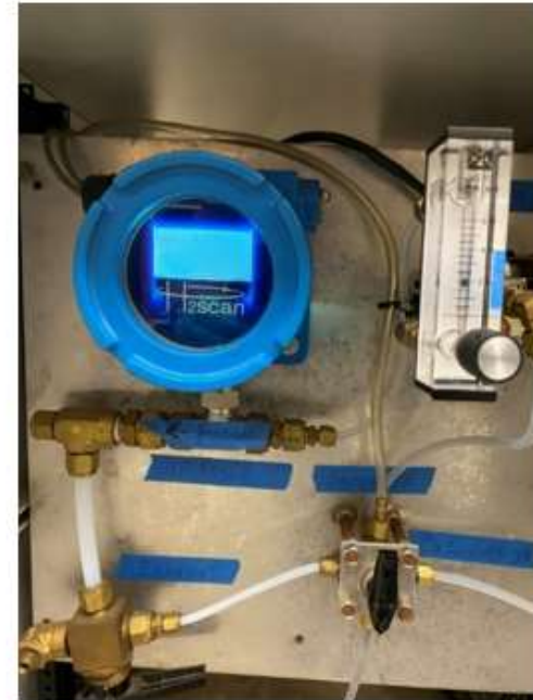
H2Scan Hydrogen Analyzer Sample System
