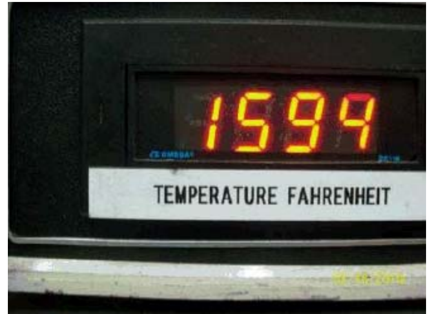
Burner Temperature at 1594°F
