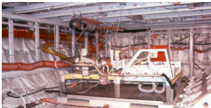
Figure 3. System Installed in A320 Cargo Bay
