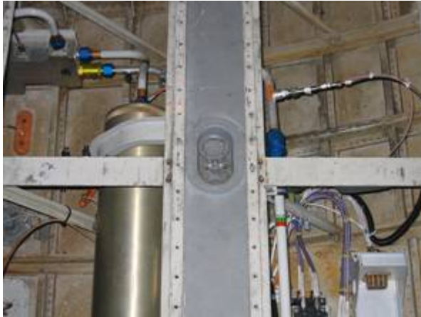
Inerting Distribution Line Probe
