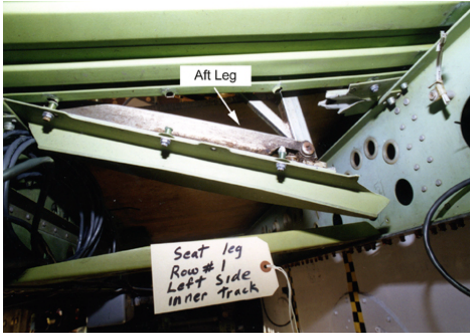
FIGURE 27. DISPLACEMENT OF INNER SEAT TRACK INTO CARGO AREA
