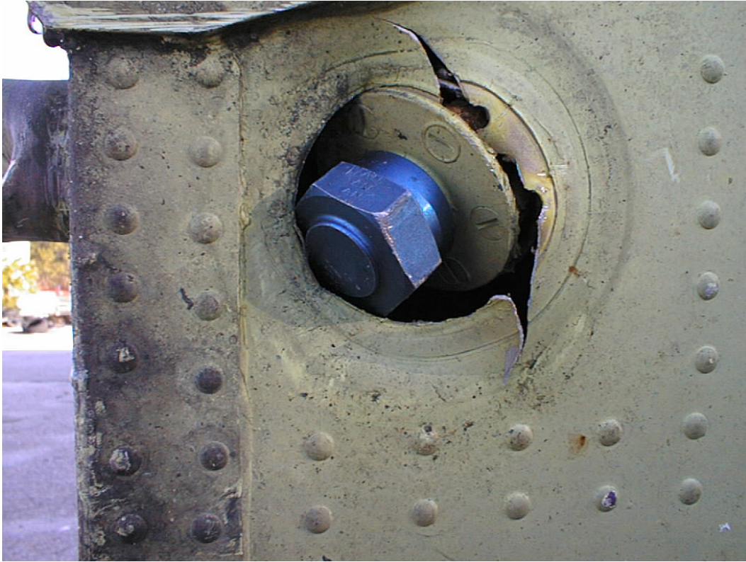
FIGURE 19. CRUSHED GRAVITY FEED OUTLET IN CELL 4
