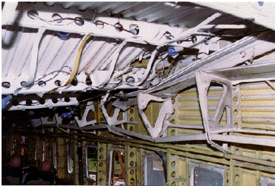
FIGURE 34. CEILING DEFORMATION POSTTEST COPILOT SIDE
